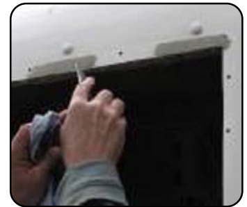
Putty tape being applied to the dished-in area of the fiberglass. The rag is used to dampen the putty surface with paint thinner to keep the knife from sticking.
