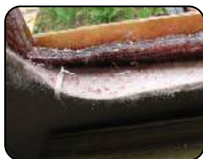
"Rat fur" and insulation pulled back with the rivets and window removed
