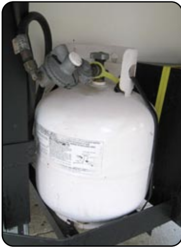
Propane tanks and valves should be checked and maintained annually.
