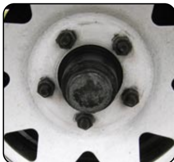
Wheel bearings need to be checked and serviced every year.
