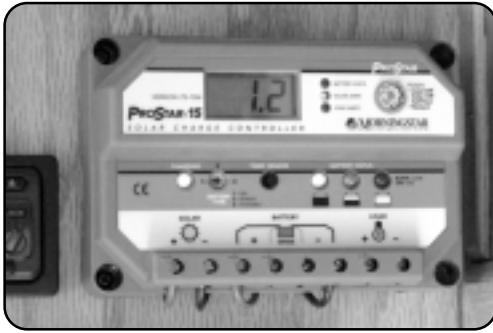
The ProStar-15 controller was mounted over the wardrobe right next to the radio.
