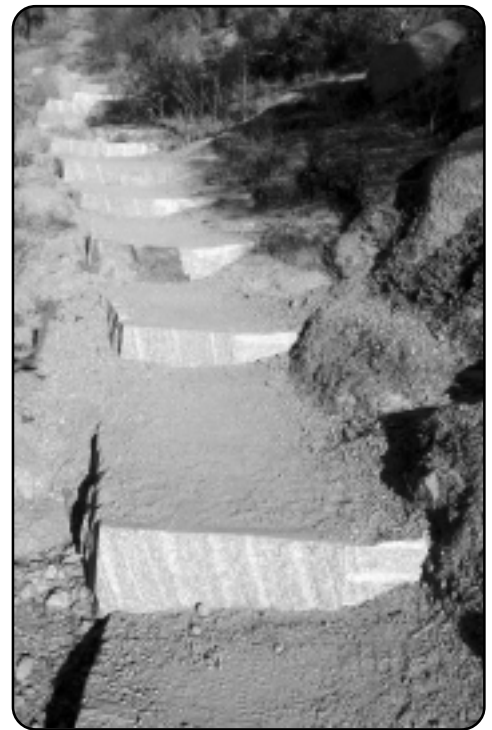
Hiking is made easy on some of the trails as hundreds of cut granite steps have been placed on the steeper parts
