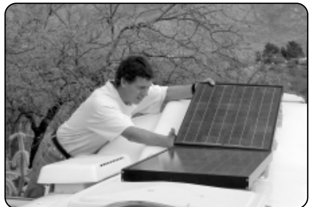
George Villec of GeoInnovation installing the solar panels on Scamp 1 in Tucson, Arizona.
