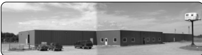
Scamp-Eveland, Inc's new production building was well along in July - the outside was mostly complete while work continued on the interior. Scamp hopes to resume production within a few months.
