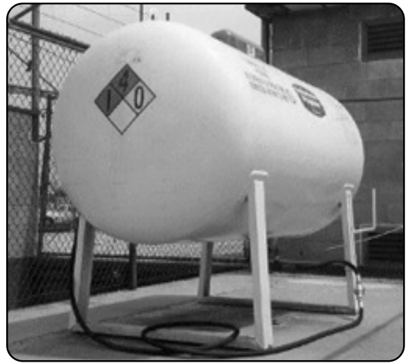
Typical large propane storage tank at a supplier.
