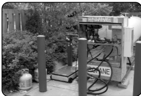
Fueling Station – This typical propane filling facility has a relatively large storage tank, pump, hoses, and even the old fashion scales for servicing small tanks. Safety guard posts and a couple 20-pound tanks are also visible.
